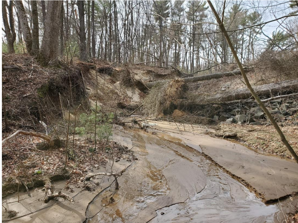
Erosion in Spring Park
